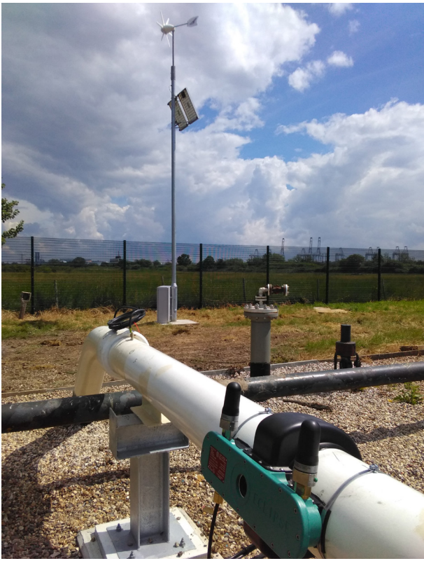
Figure 3. Atmos Eclipse installed at a tank farm with wind and solar power.
