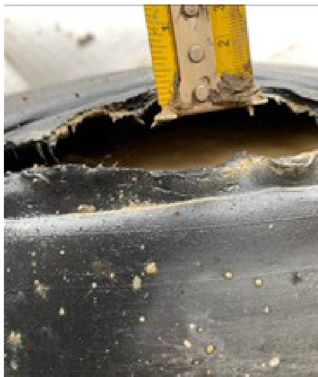
Figure 2. The failure point of this customer's pipeline was roughly 14 in. long.
